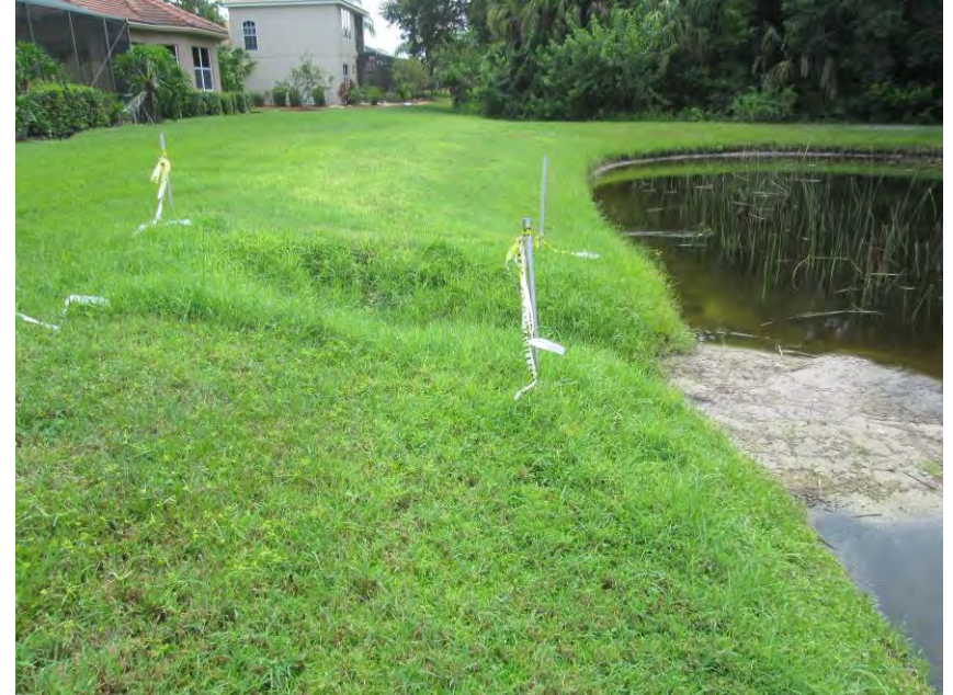
Swale erosion on east side of pond 14
