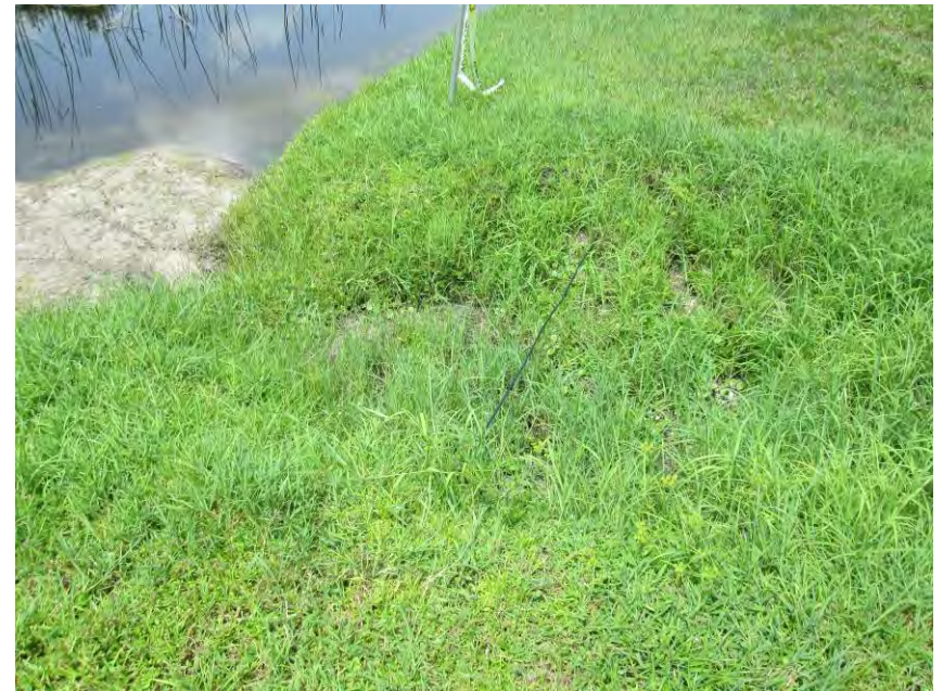
Swale erosion on east side of pond 14
