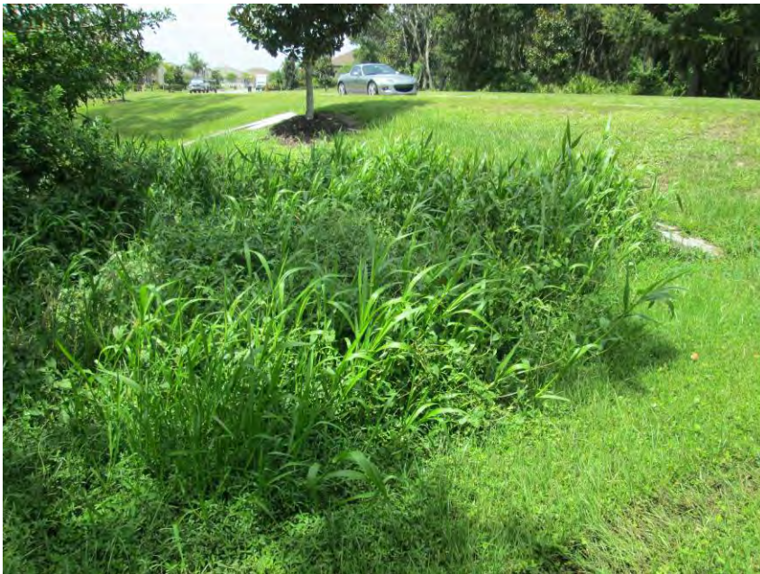
Southeast side of Goldenrod Ave- clear 40'x10' of vegetation in channel
