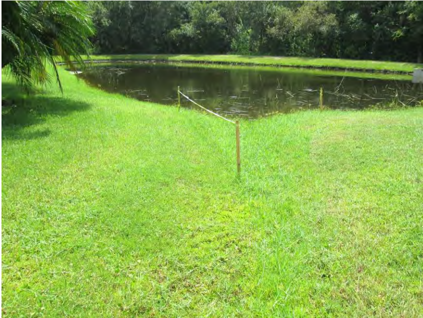
Swale erosion on northeast corner of pond 14
